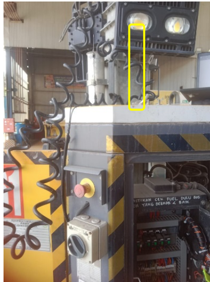
Figure 3. Placement of GPS antenna and LTE antenna on Tower Lamp
